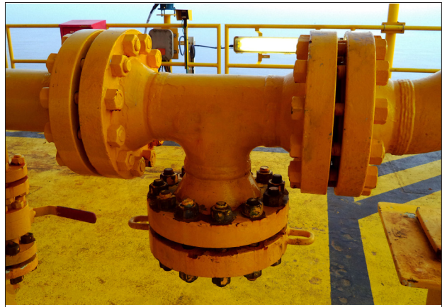
Figure 2. Approximately 90 percent of produced water is managed by underground injection using pipes such as those pictured, which are connected to deep injection wells. Credit: Mr. PK via Shutterstock
